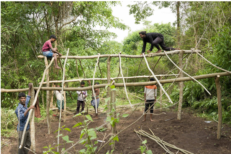
Jenu Kuruba families begin to construct a house for their ancestors, as they rebuild their old village inside Nagarhole National Park. © Sartaz Ali Barkat/ Survival
